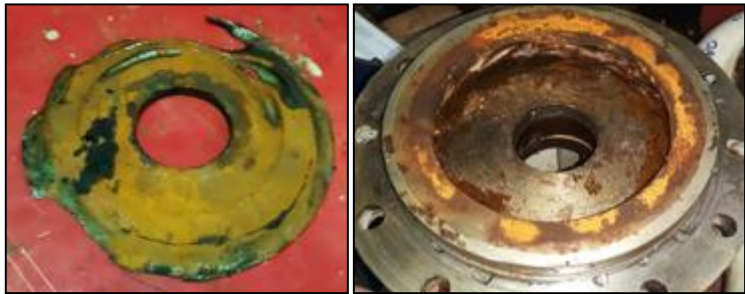
Figure 2. Damage that occurs to the pedestal cover and pedestal (Documentation PT. XYZ)
